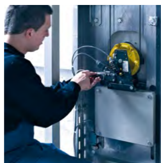
Service for elevators
