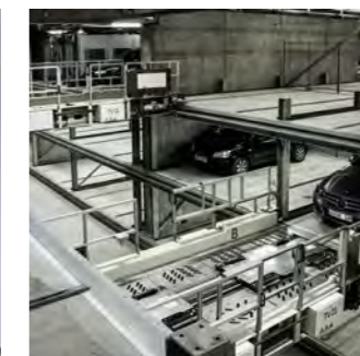
Fully automated car park system CUBILE® (Aarhus)
